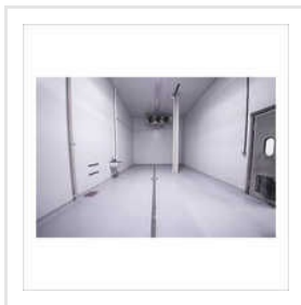
Carrier Cold Storage Room
