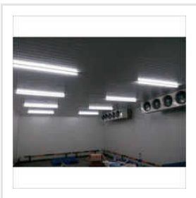
Dairy Products Cold Storage Room
