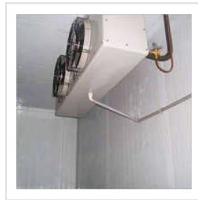
Automatic Cold Storage Room
