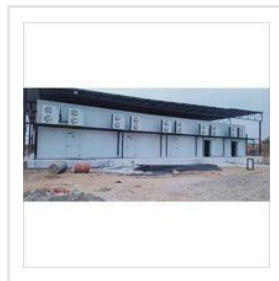
Mushroom Cold Storage Plant
