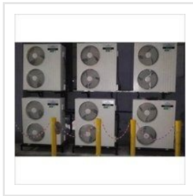
Cold Room Outdoor Unit
